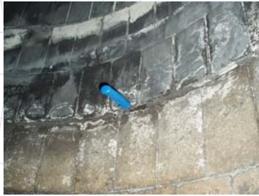
Damaged joints in a venturi
