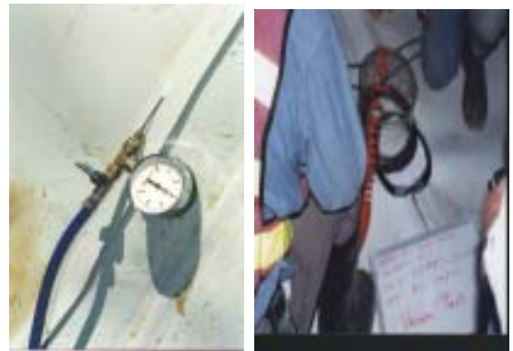
Seam Testing using air pressure for double seams and vacuum box for extrusion seams
