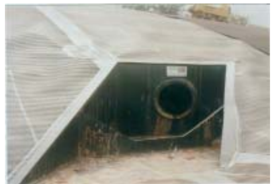
Pipe Penetration (Frank/Sansenh_04)
