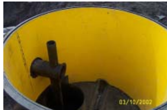
Leachate collecting manhole out of HDPE
