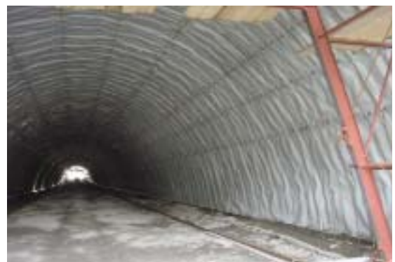
View on finished tunnel section (prior to installation of inner shell concrete)
