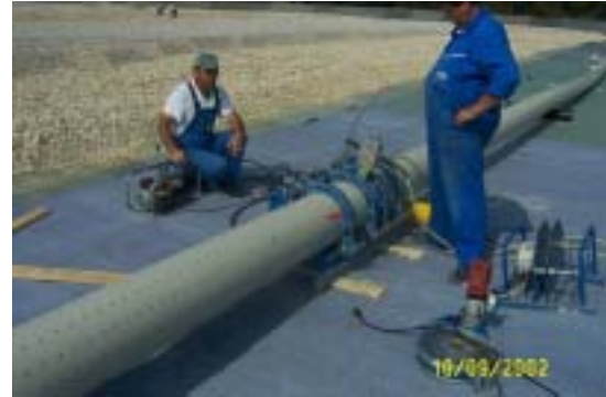
Drainage pipe out of PE
