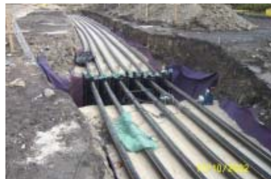
Leachate collecting pipe systems out of HDPE
