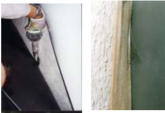
The AGRUFLEX tunnel liner is manually welded to the discs by hot gas welding
