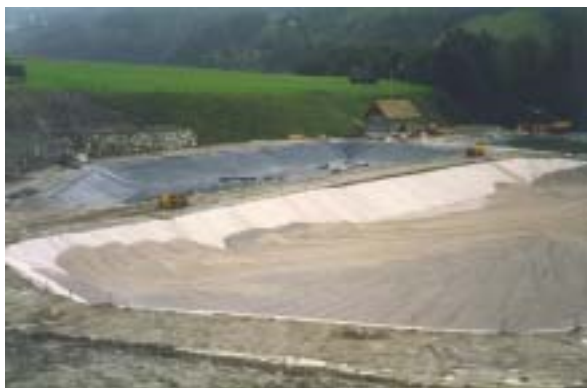
Biological Treatment pond
