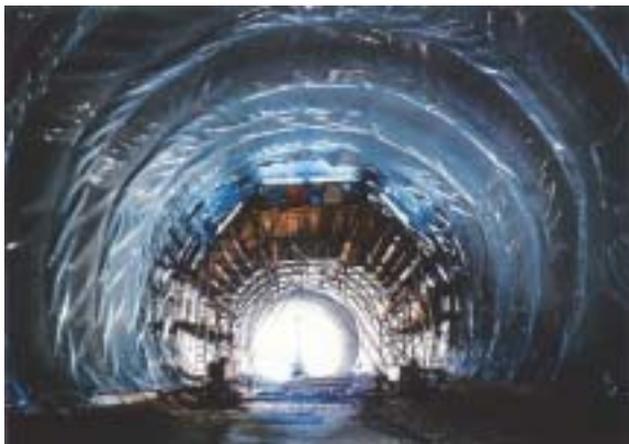
View on scaffolding for installation and welding of the AGRUFLEX tunnel liners
