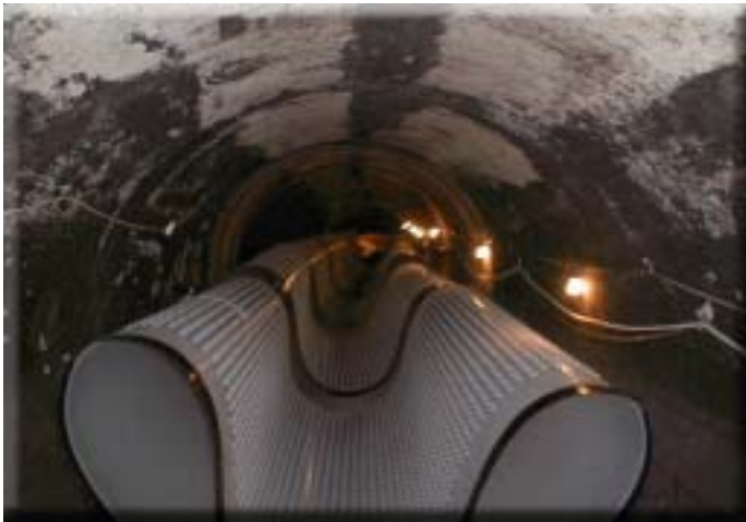
Transport des Inliners in das bestehende Rohr Transport of Inliners into the existing pipe
